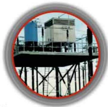
Substation, Platform, Mexico
